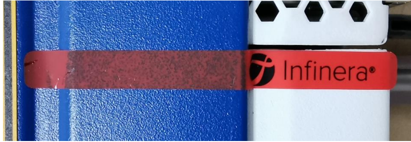
Figure 4 – Tamper-evident label: intact
