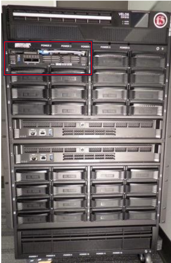
Figure 7 – VELOS CX1610-BX520 tested blade (in blade slot #1-2) -delineated with a red rectangle- mounted on the chassis equipped with 30 blanks/ filler panels.
