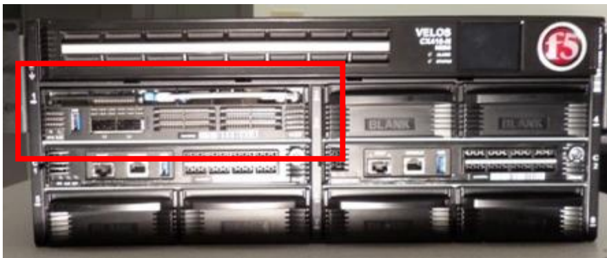
Figure 8 – VELOS CX410-BX520 tested blade (in blade slot #1-2) -delineated with a red rectangle- mounted on the chassis equipped with 6 blanks/ filler panels.
