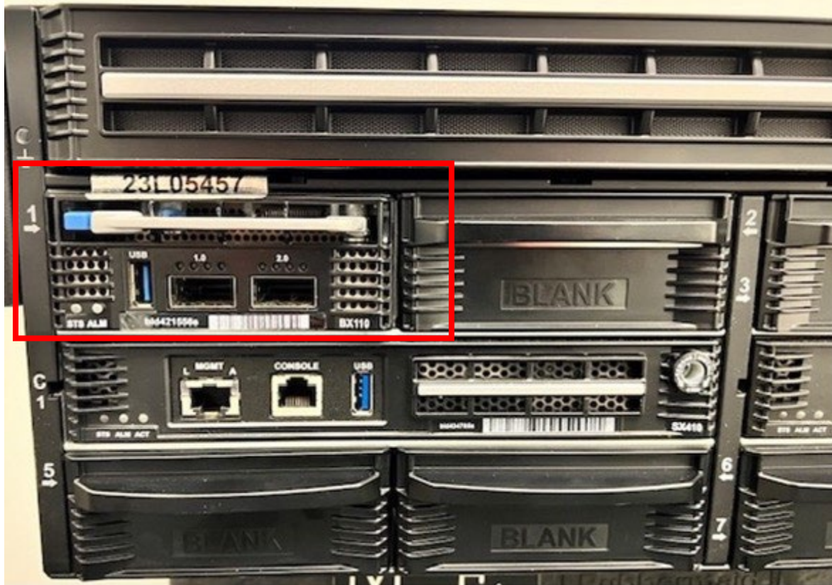
Figure 11 – Tamper labels on VELOS CX410-BX110 blade mounted on chassis. The tamper label affixed between blade and chassis is positioned to provide evidence if the tested blade in slot #1 is removed from the chassis.
