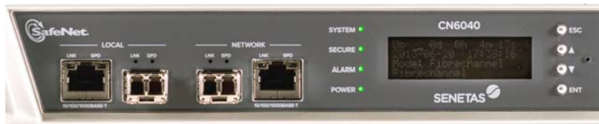
Figure 16 – A6040B 1G Ethernet ports close-up - SFPs installed
