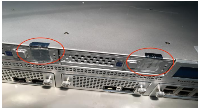
Figure 5 – EX-9000 Tamper Seals #6 and #7 - Front Drive Bays
