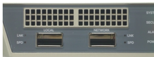
Figure 13 – A9120B 100G Ethernet ports close-up – QSFP28s not installed
