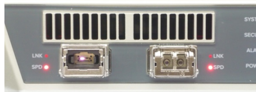
Figure 12 – A9100B 100G Ethernet ports close-up - CFP4s installed
