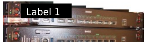
Figure 19 - Tamper labels on VIPRION B4450 in chassis (1 of 5 tamper labels shown)
