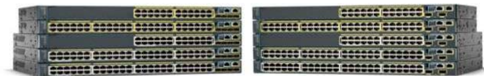
Figure 3: Cisco Catalyst 2960-S Series Switches
